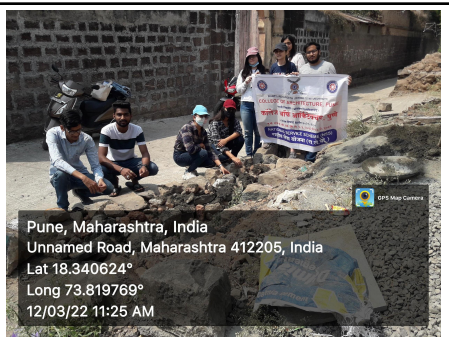
ACTIVITY :- NSS VOLUNTEERS and students are helping to construct a stone masonry, boundary wall.
